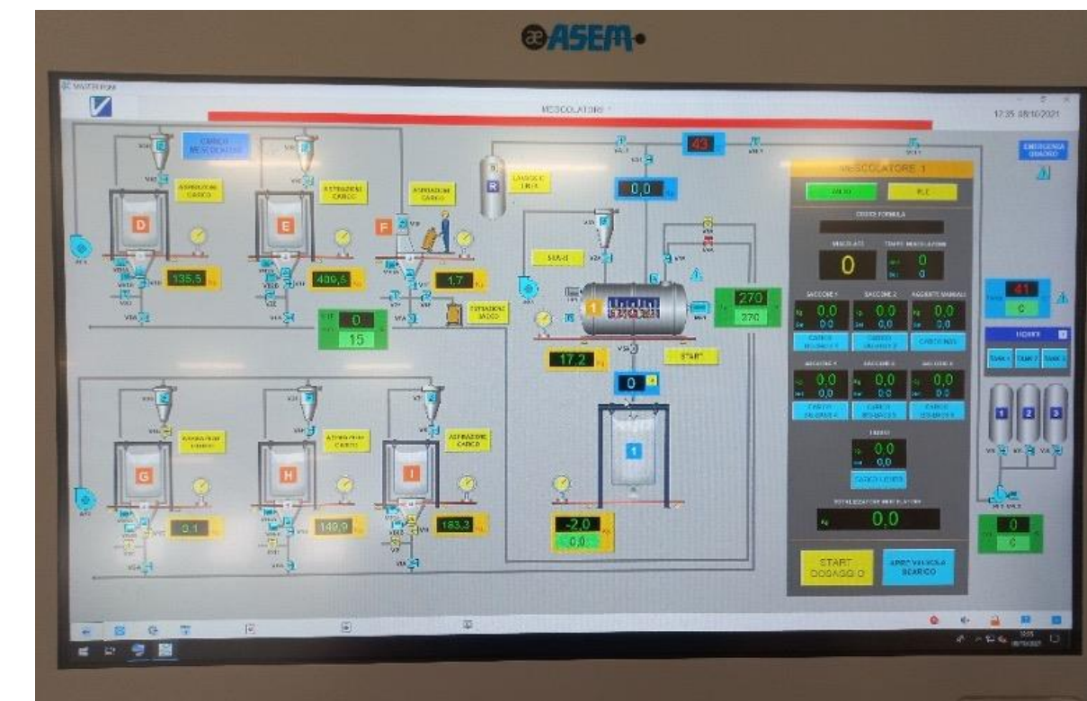
Pneumatic Conveyors system monitoring
